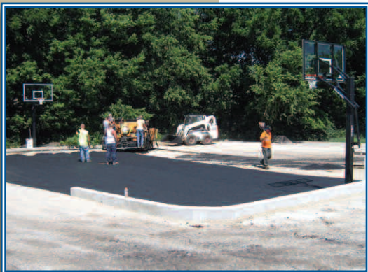
The new basketball court in the parking area was installed this summer.
