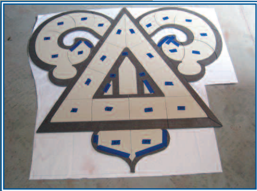
A brand new foyer inlay was installed this summer along with new paint.
